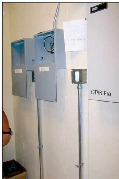
FIGURE 2. A BAS, installed to monitor energy consumption, provides real-time and trending data to track and compare energy use over time.
