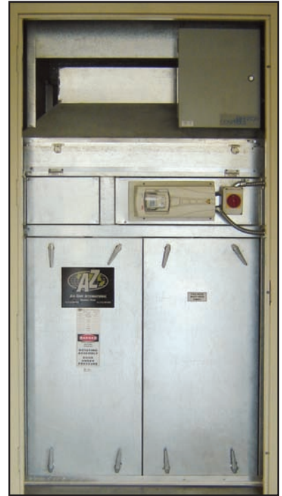
FIGURE 3. Air column fans are installed inside the building to maintain the underfloor air plenum pressure.
